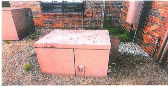
OLD CENTRAL RECEIVING TRANSFORMER & PAD
