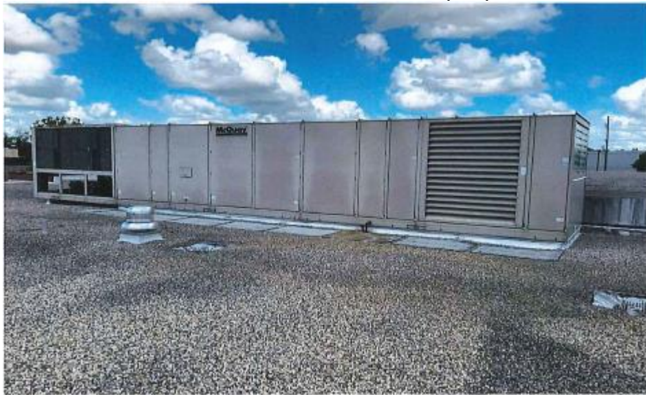
NEW BALTIMORE ROOFTOP UNIT (RTU)
