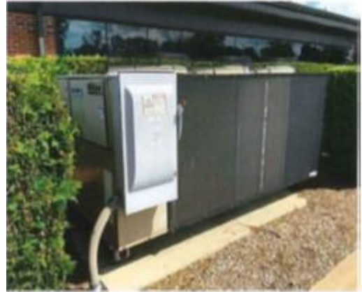
AIR CONDITIONING CONDENSER UNITS
