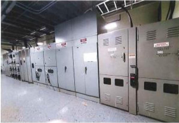
COURT BUILDING ELECTRICAL SUBSTATION, SWITCHES, PRIMARY FEEDS
