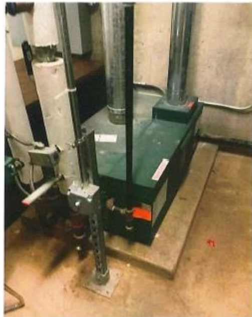
NEW BALTIMORE – BOILER 2
