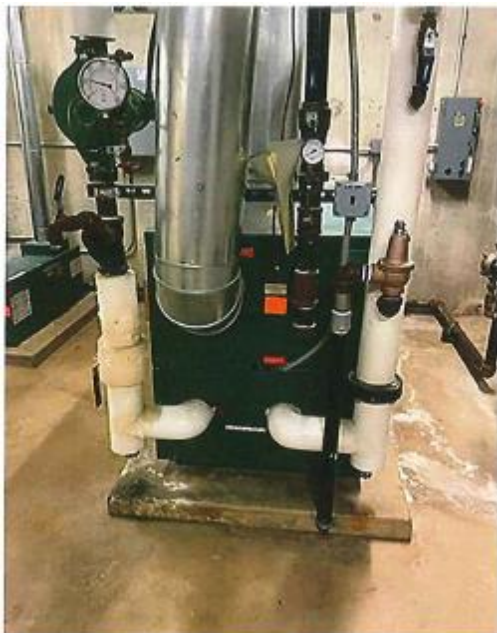
NEW BALTIMORE – BOILER 1
