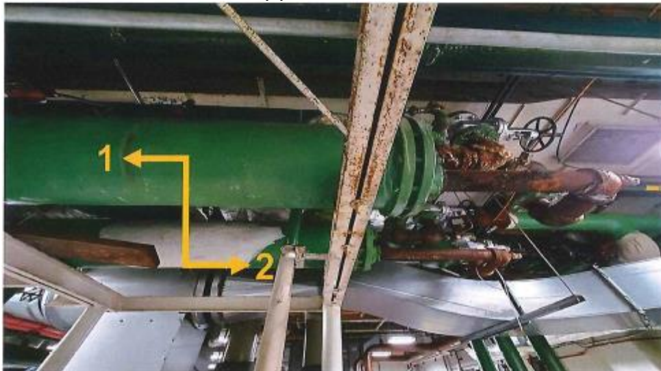
TWO (2) HEAT EXCHANGERS
