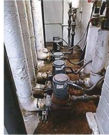
COUNTY BUILDING PUMPS
