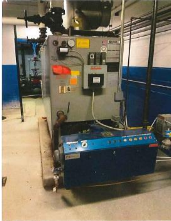
HALL ROAD WAREHOUSE BOILER
