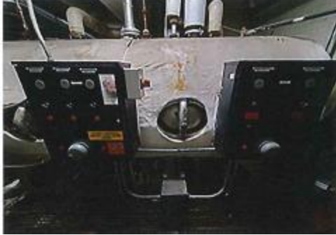
COUNTY BUILDING CONDENSATE RECEIVER
