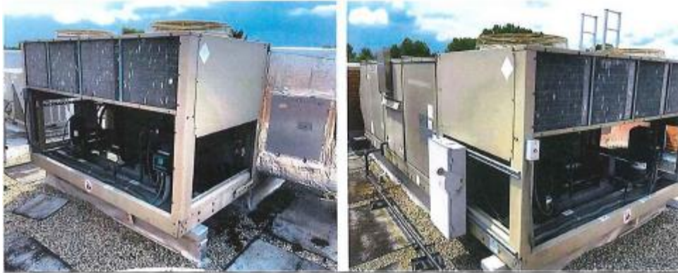
MEDICAL EXAMINER ROOFTOP UNITS
